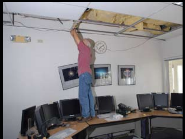
Facilities Senior manager Dennis McBride assesses damage at headquarters. A stopped clock shows when the 6.7 magnitude quake hit.
